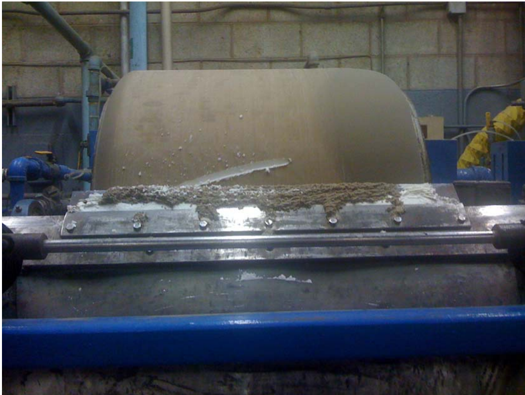
Figure 20: Alar RVF Filtration with FW40 precoat filteraid
