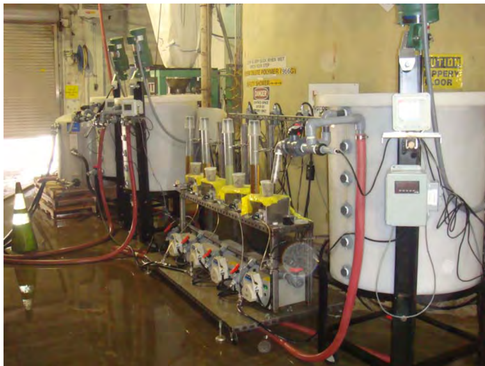
Figure 5: ADM Decatur Nickel Removal pilot plant (5/13/2011). Four 100 gal reactors.
