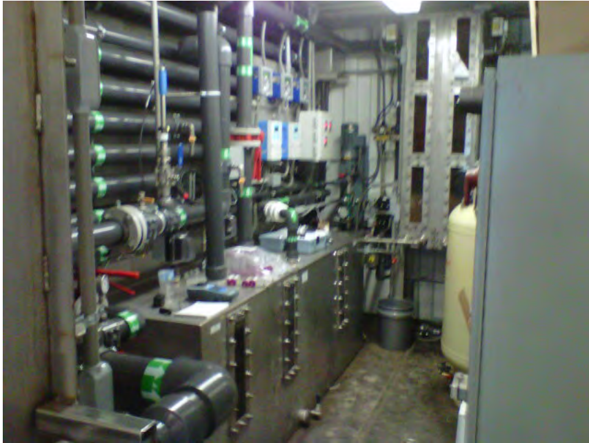
Figure 18: Krofta Sand Filter at ADM pilot plat
